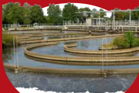
Waste Water Treatment
